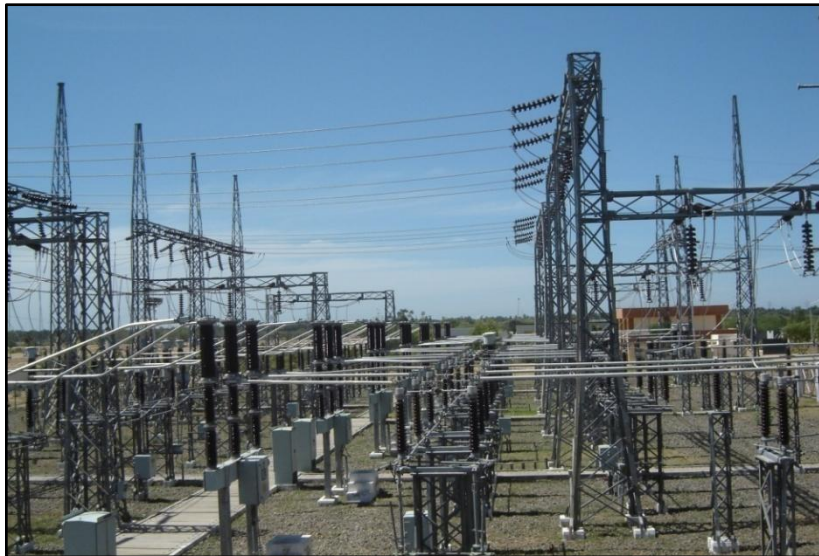
95 MW CCPP Substation, Valathur, Tamil Nadu
