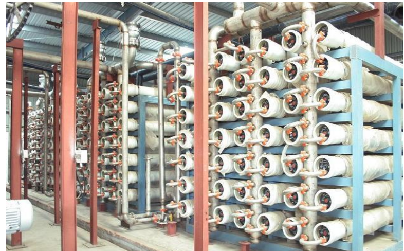
Effluent Treatment Plant – RO System Veerapandi
