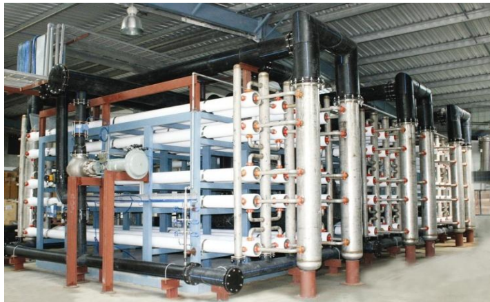
Effluent Recycling Plant - Tiruppur
