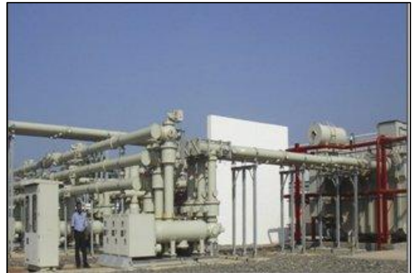
230/ 11kv Gas Insulated Substations Substation, Hyundai , Chennai
