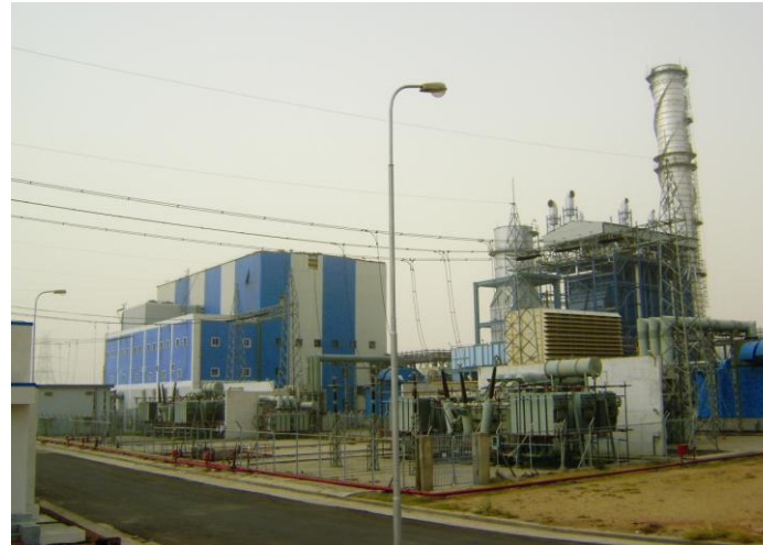
330 MW CCPP RRVUNL, Dholpur, Rajasthan
