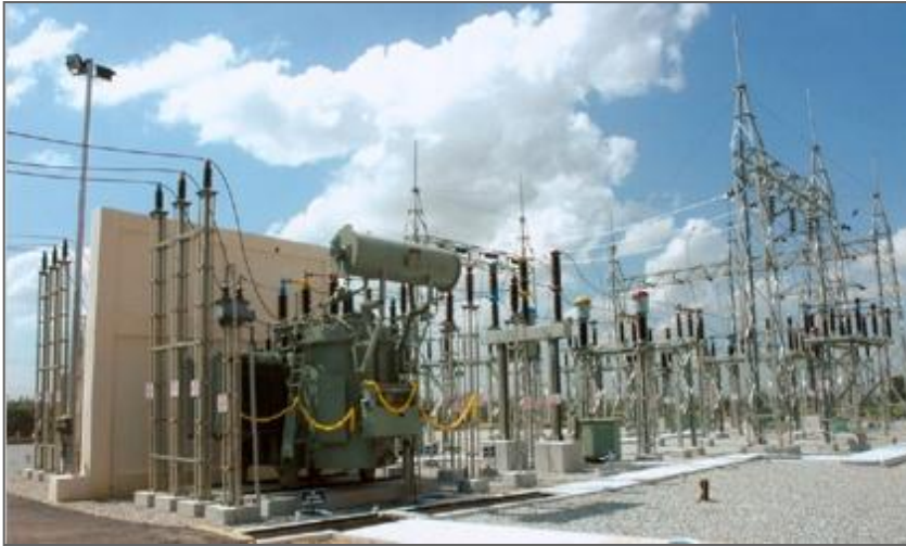
66/11 KV KPTCL Substation, Ganji Kunte
