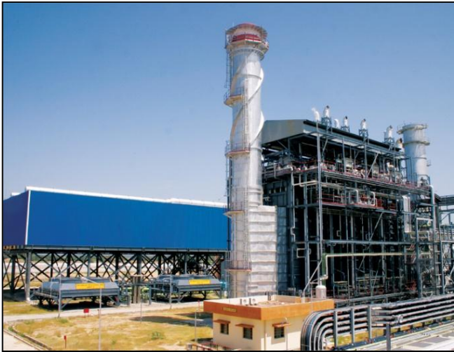
95 MW CCPP Valathur (Phase I), Tamil Nadu
