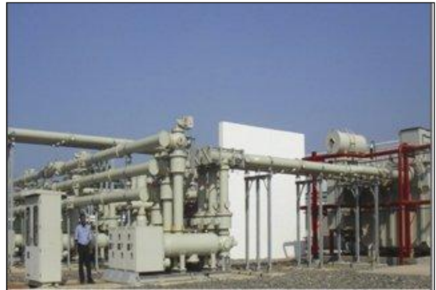
230/11 KV Gas Insulated Substations, Hyundai, Chennai
