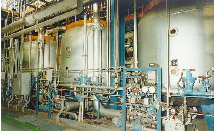
CPP – Condensate Polishing Plant
