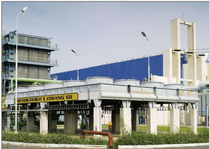
Air Cooled Heat Exchanger, 120MW CPP Karuppur, Tamil Nadu
